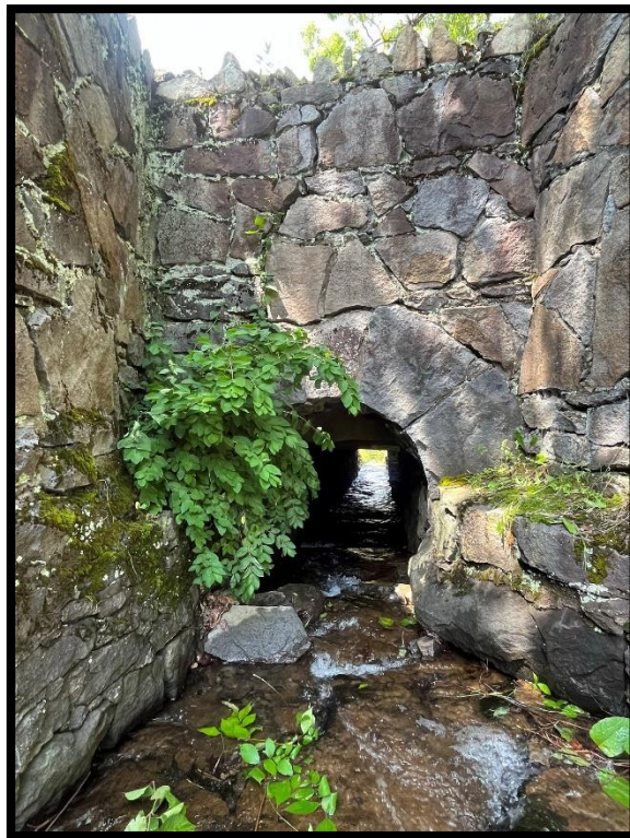
Photo 3.4.2 Stone culvert at the Marine Corps League Museum which was built in 1936 by the Works Progress Administration.
