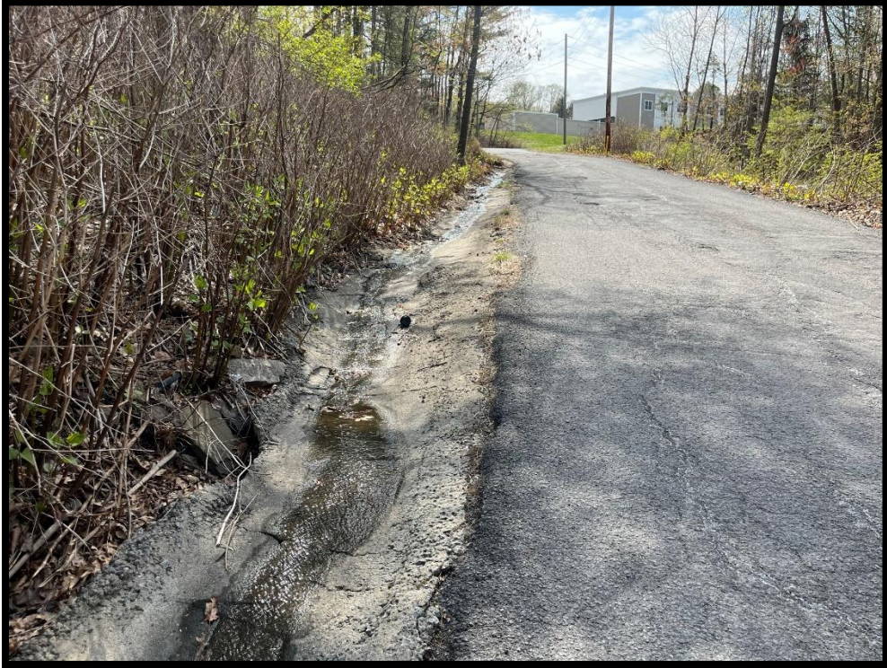
Photo 3.7.7 The concrete gutter along the Nursing Home driveway is insufficient to convey flow from larger storm which results in flooding of the cartway.
