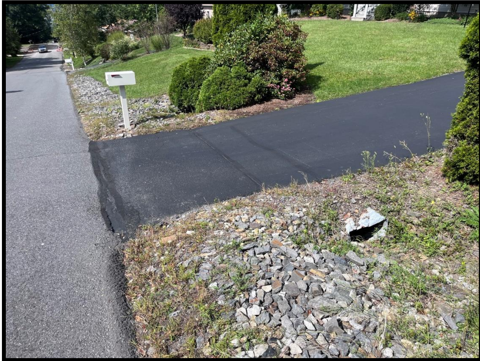
Photo 3.2.9 The water then flows through the stone shoulder until it hits an obstruction, such as a driveway crossing, which deflects the water back into the roadway.
