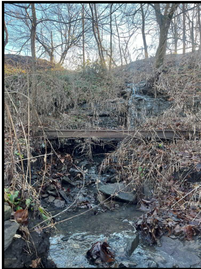
Photo 3.1.2 Stormwater runoff from East Mountain has eroded ditches through the abandoned railroad grade which is located between Moltke Avenue and Route 81.
