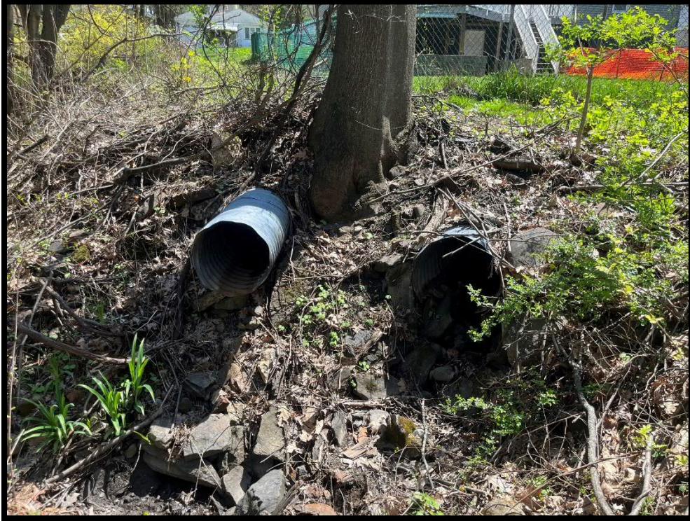
Photo 3.8.3 The existing Florida Avenue drainage system discharges into the woodland behind 120 Florida Avenue.
