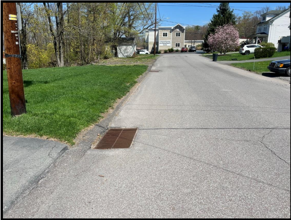
Photo 3.8.2 These two stormwater inlets have been insufficient to eliminate the ponding of stormwater in a low-lying section of Florida Avenue.
