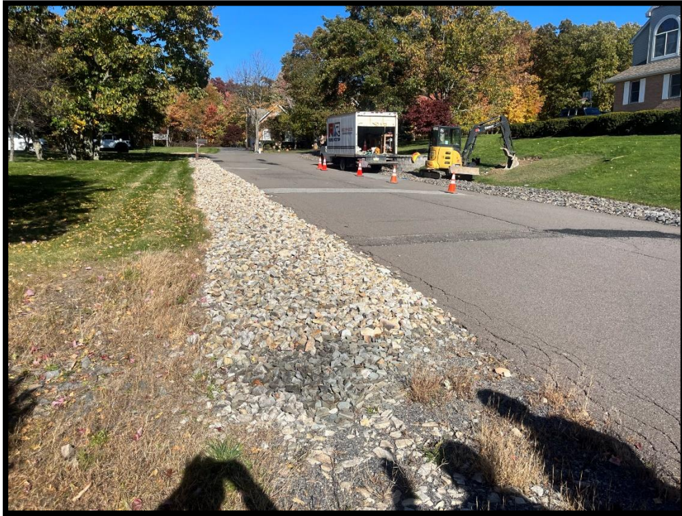
Photo 3.2.5 It appears that roadway runoff drains into the stones along the roadway shoulder and is then unable to drain into the inlets.
