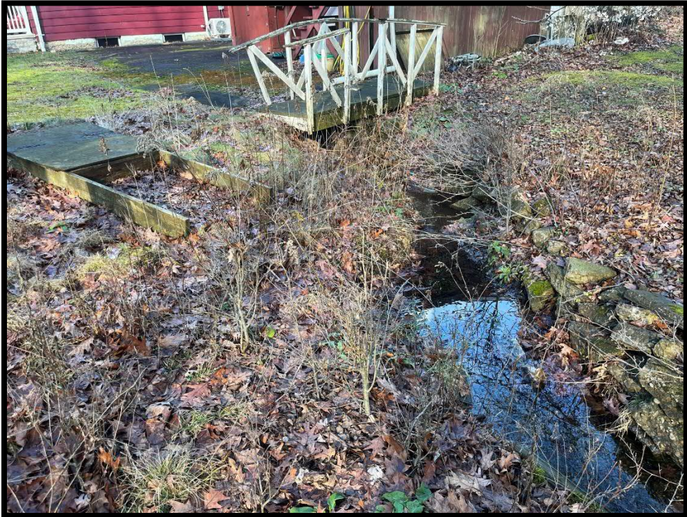
Photo 3.6.3 The existing stormwater inlet for this drainage system is located under this small bridge.
