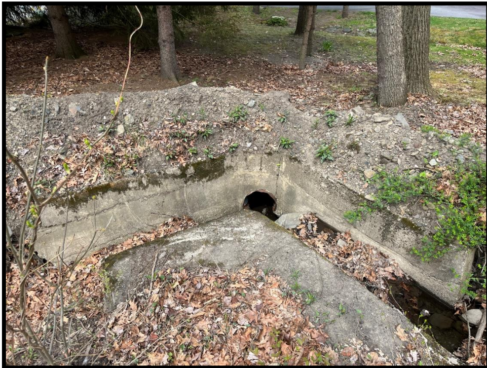
Photo 3.7.6 This is the existing driveway culvert below Ariel Street. It is both undersized and in disrepair.
