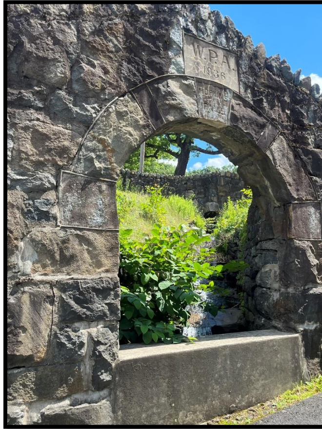
Photo 3.4.3 Stonework at the Marine Corps League Museum which was built in 1936 by the Works Progress Administration.
