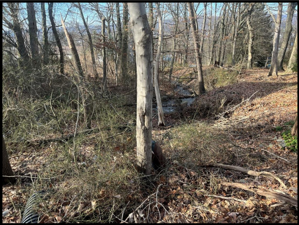
Photo 3.4.5 The culvert discharge below Wintermantle Avenue needs to be improved with stabilization and a better defined channel.
