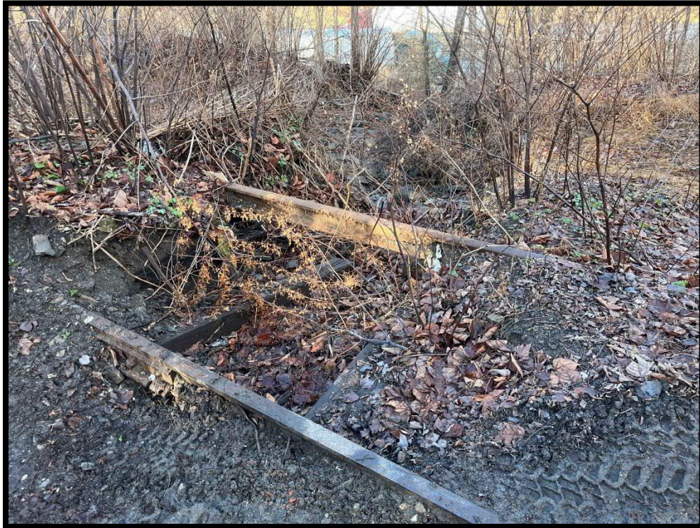
Photo 3.1.5 The unregulated flow of stormwater runoff flows directly towards Route 81 where it has caused dangerous flooding in the past.
