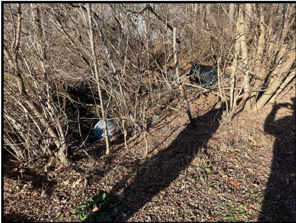
Photo 3.5.4 The existing discharge below Wintermantle Avenue should also be stabilized.
