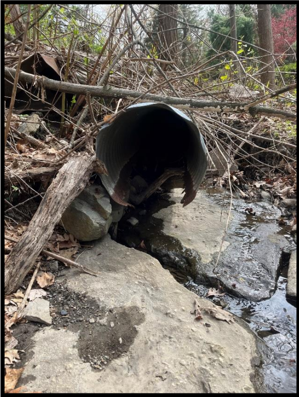
Photo 3.7.5 The downstream end of the driveway culvert shows the structural failure of the corrugated metal pipe.
