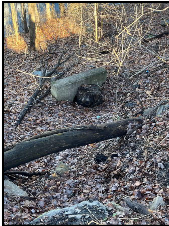
Photo 3.1.6 Lack of maintenance of PennDOT drainage structures has also been responsible for flooding on the highway.
