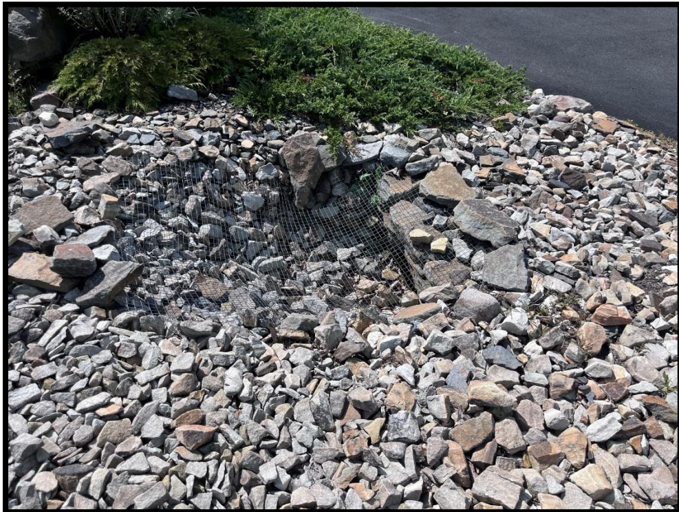
Photo 3.2.10 Each inlet should be opened up and existing debris and silt should be removed.
