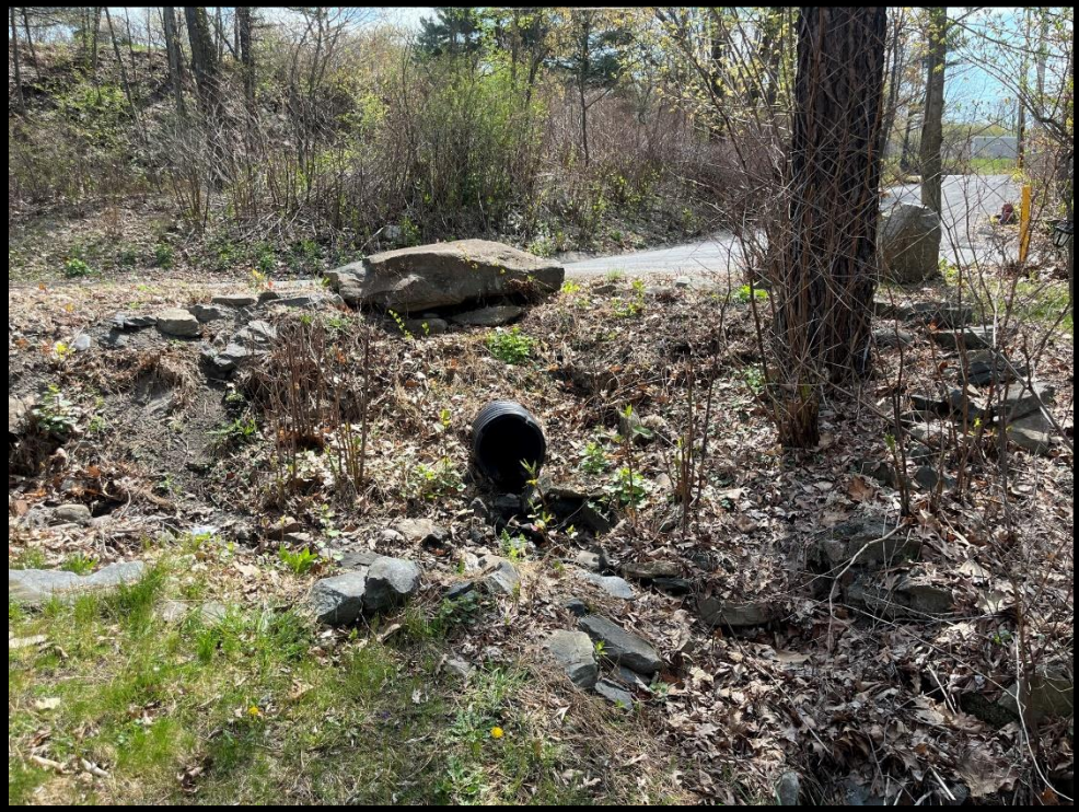
Photo 3.7.9 Discharge from the Linwood Avenue culvert has no outlet protection or downstream drainage swale .
