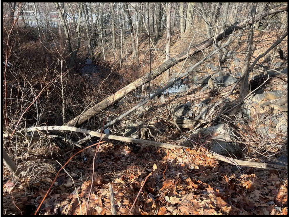
Photo 3.4.7 The channel below Moltke Avenue should be cleared of debris to improve flow.
