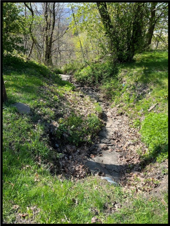
Photo 3.3.8 Stabilization is also needed in the channel flowing downhill from the end of East Elm Street.
