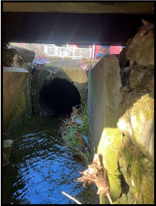
Photo 3.6.4 Existing headwall draining stormwater runoff into the drainage system behind the homes on East Mountain Road.
