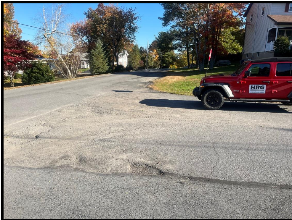
Photo 3.9.6 The new drainage system will also alleviate flooding at the intersection of Batluck Street and Seymour Avenue.
