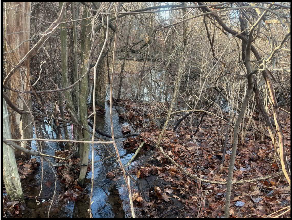
Photo 3.4.8 The culvert under the railroad has failed and water now ponds above the rail line until it reaches a level where it over-tops the grade.
