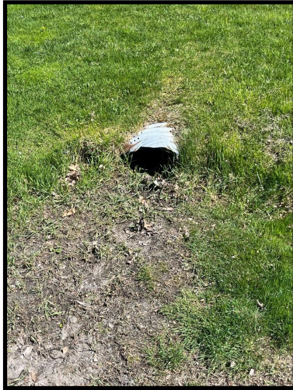
Photo 3.3.9 The existing storm drain on the northern side of East Elm Street should also be replaced since the current corrugated metal pipe has failed.
