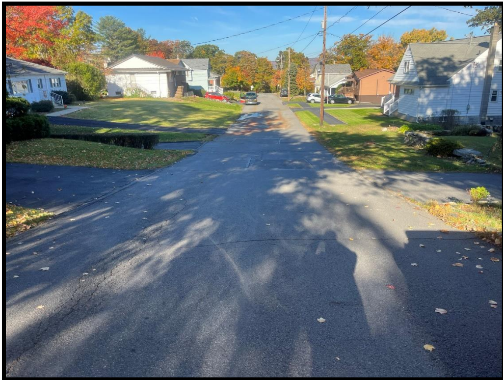
Photo 3.9.4 View looking down Snooks Street at an area which is often flooded by stormwater runoff. Undulating topography makes it impossible to drain water away from this area without a storm sewer system.
