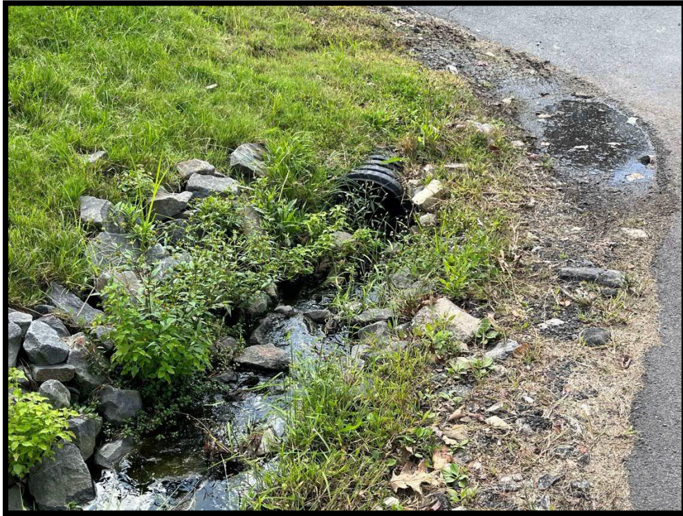
Photo 3.3.3 The lack of a headwall at the inlets at Derby Avenue allows runoff to bypass the storm drains and run down East Elm Street.
