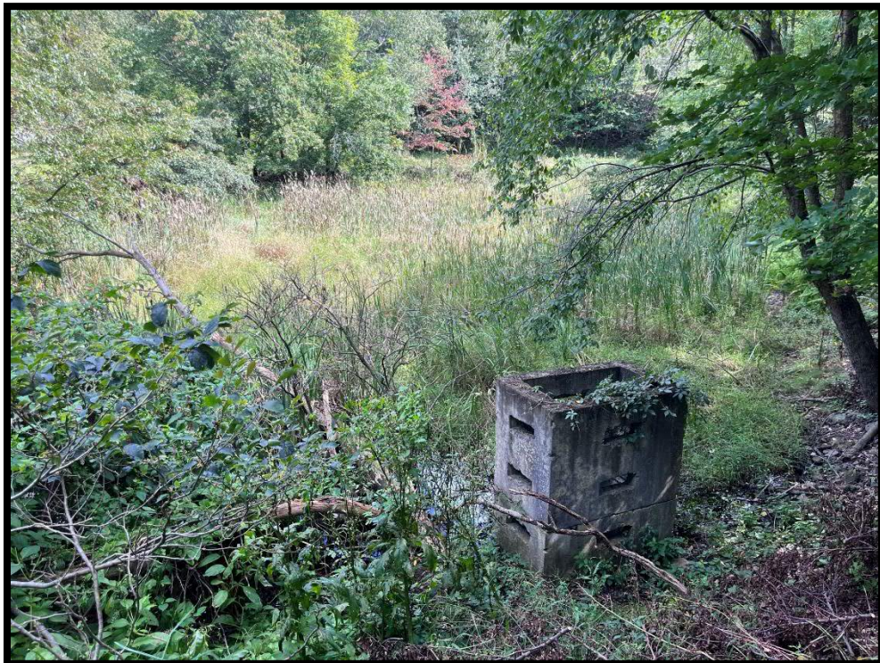
Photo 3.2.2 View of the existing stormwater detention basin which was built as part of the Mountain Laurel Estates Subdivision.
