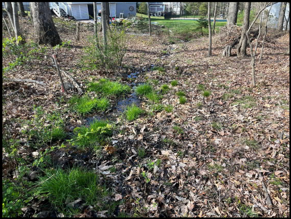
Photo 3.9.2 Groundwater seepage flows around areas filled for construction of the new homes on Grande Circle.
