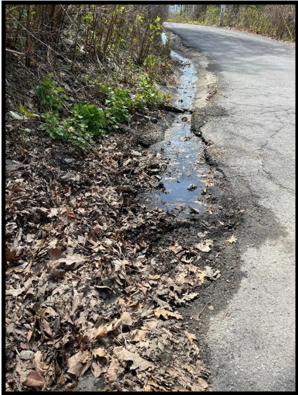
Photo 3.7.8 Inlet for the cross drain under Linwood Avenue is filled with silt and debris, and not functioning.
