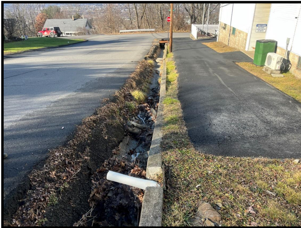
Photo 3.5.2 View looking down Beech Street from Blucher Avenue. Flooding and icing conditions pose a hazard to vehicles coming down the hill.
