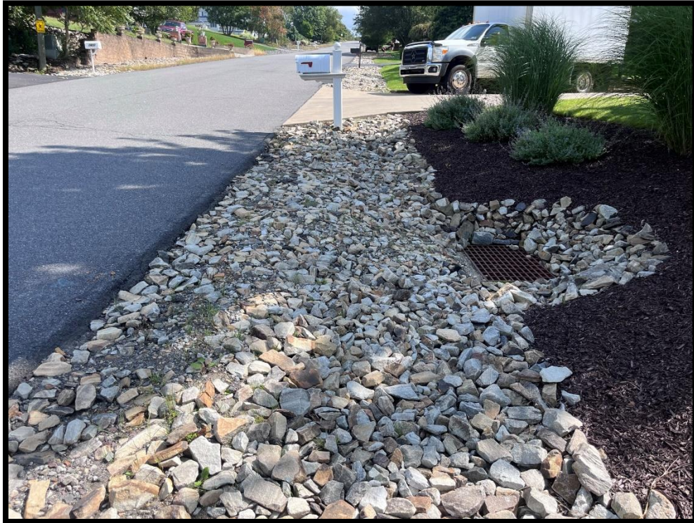
Photo 3.2.7 To correct the current drainage problems along Cherry Street, we recommend adding a paved apron from the cartway to the inlets.
