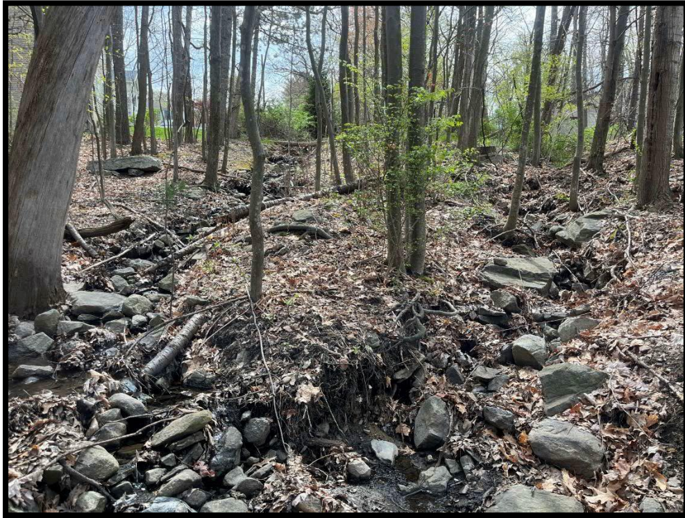
Photo 3.7.5 View of the unstable conditions that have developed within the drainageway of the Ariel Street stormwater runoff.
