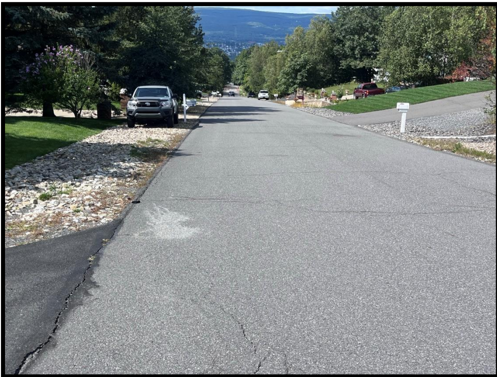
Photo 3.2.4 Existing stone shoulders on both sides of Cherry Street have created a drainage problem along the roadway by keeping runoff from entering the inlets.
