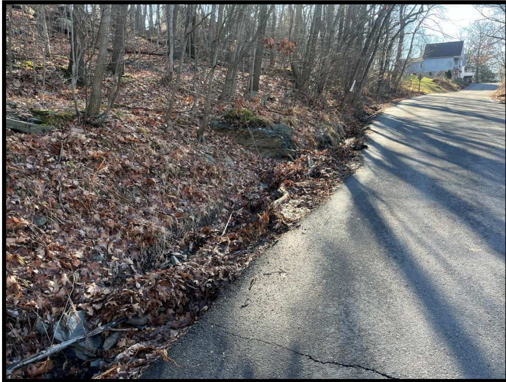
Photo 3.5.3 This drainage swale along Blucher Avenue should be excavated and stabilized to better handle stormwater runoff.
