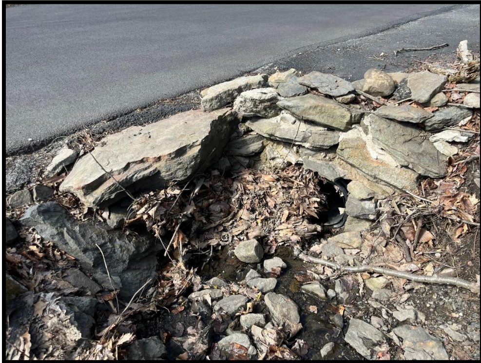
Photo 3.3.5 The culvert under Wintermantle Avenue is currently undersized and lacks proper headwalls. It is also prone to clogging by debris.
