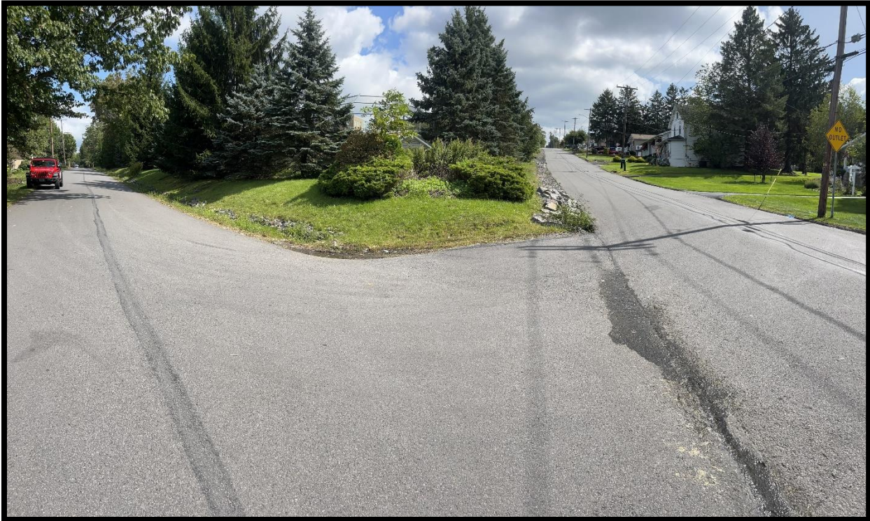
Photo 3.3.1 View looking uphill at the intersection of East Elm and Derby where stormwater runoff has been over topping the storm sewer inlets.
