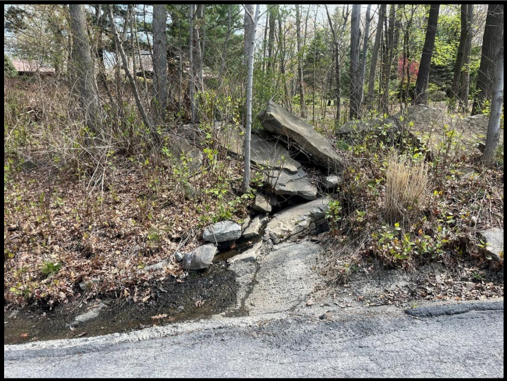
Photo 3.7.6 The swale downstream of the driveway culvert has been blocked by these large boulders.
