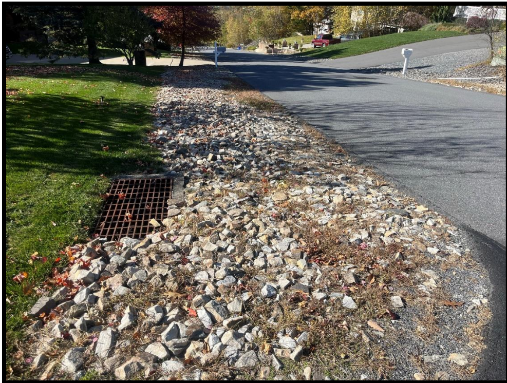
Photo 3.2.6 Stormwater inlets were placed on the back side of the stone shoulder rather than along the paved cartway
