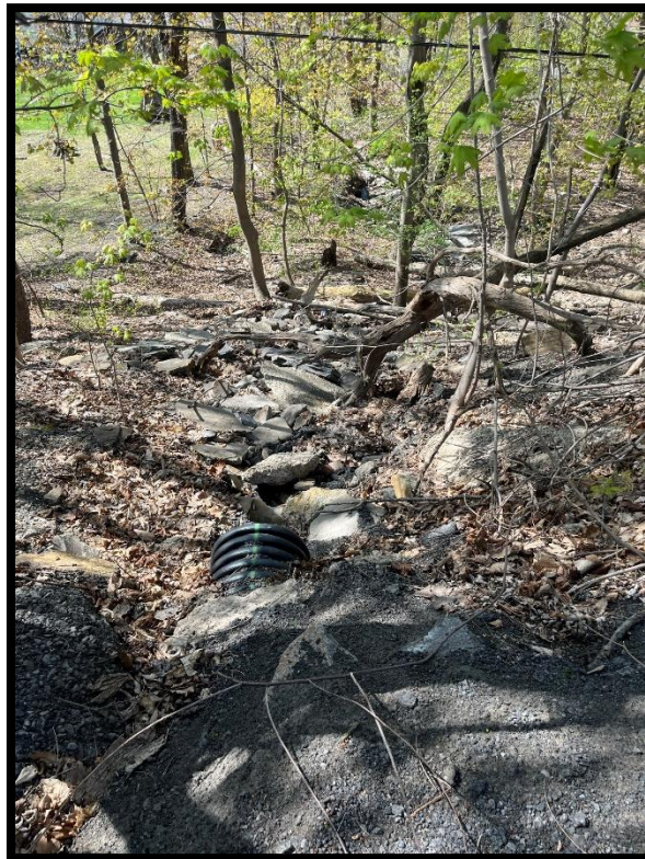
Photo 3.3.4 The East Elm storm sewer currently discharges overland below Blucher Avenue. A stabilized channel is recommended for this discharge.
