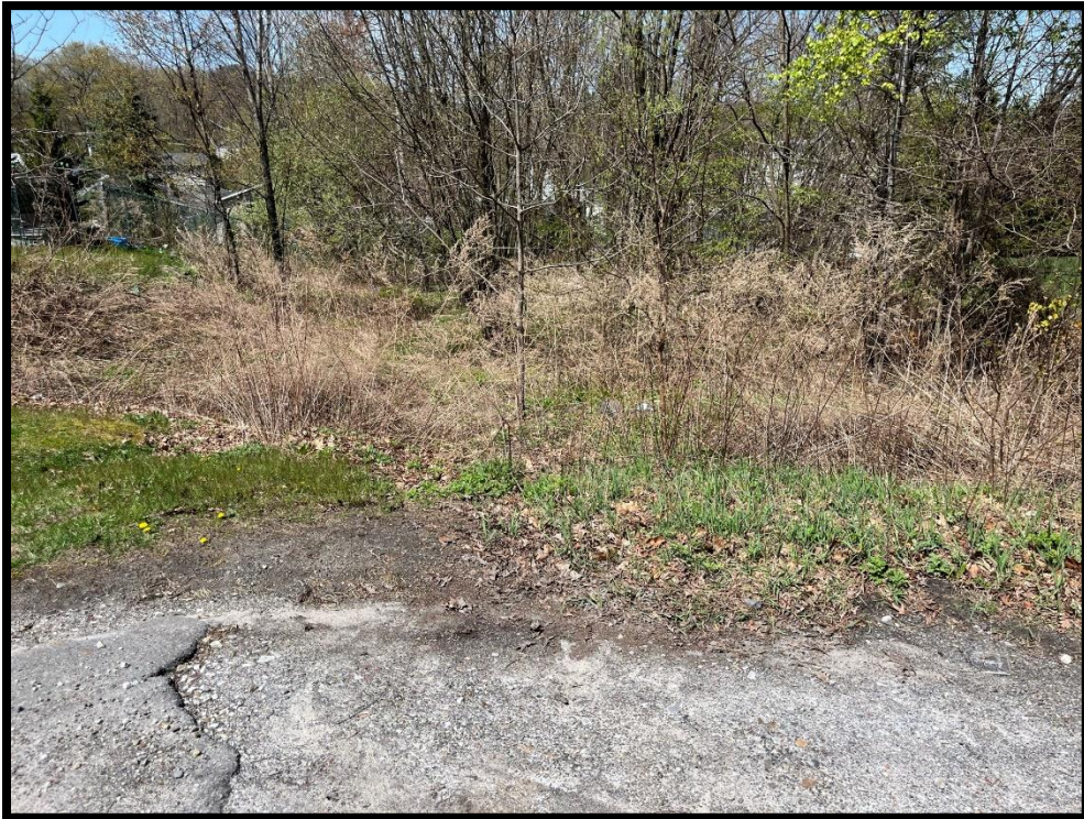
Photo 3.8.4 Missing curb along a low section on Oswald Avenue has allow stormwater runoff to bypass a catch basin on that road, and has resulted in flooding at 101 Florida Avenue.
